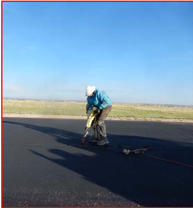
"PPRCC maintenance team member Chuck Brath, tackles several cracks on the west runway, Got cracks? Call Chuck!"
