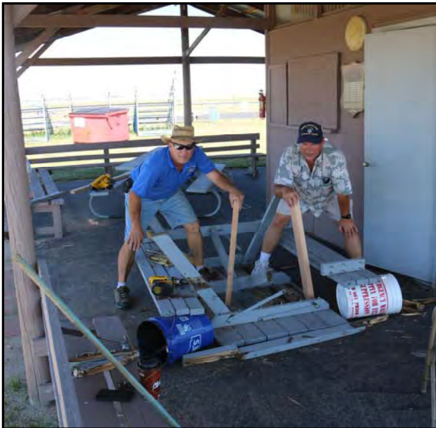
“Club members Kevin and Ed repairing one of the picnic benches days before Family Day.”
