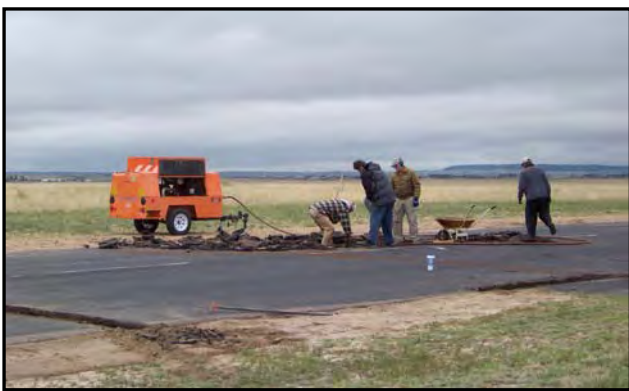
"With the help of Chuck Brath's heavy equipment, lots of the hard labor is not so hard!"
