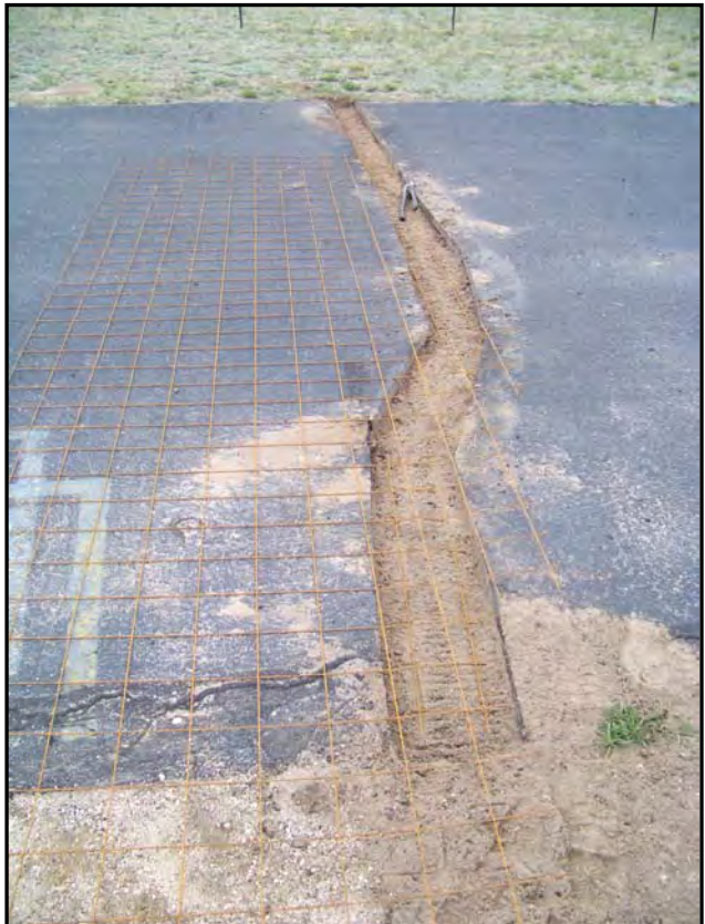
"This is one of several cracks that have been cut and cleared in preparation for cement."
