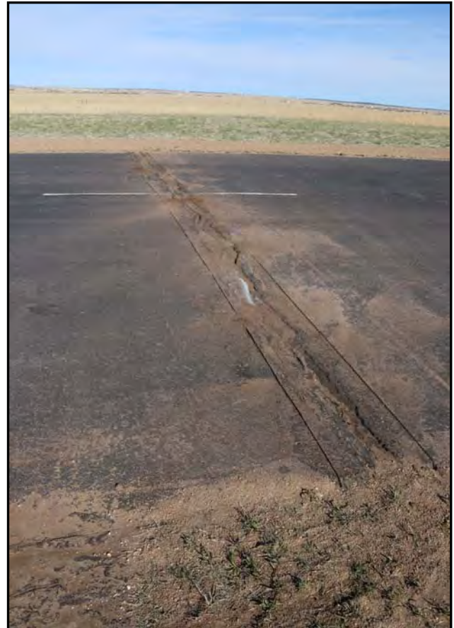
“The cuts have been made to remove the asphalt. The asphalt will then be remove and filled with cement.”
