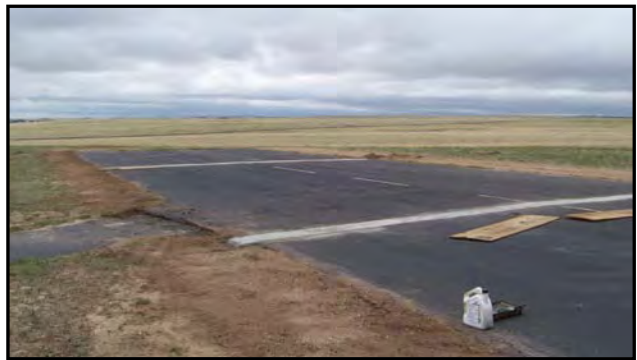
"The almost final product. The cement has been poured, it just needs to be painted black and sealed."
